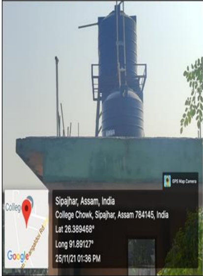
Water overflow alarm installed in all water reservoirs
