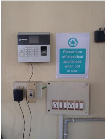
Switch off devices when not in use- a reminder
